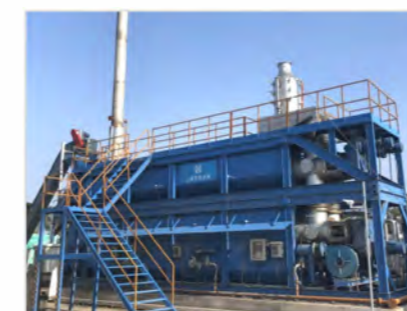
Tail gas conveying
