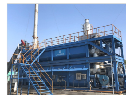
Tail gas conveying
